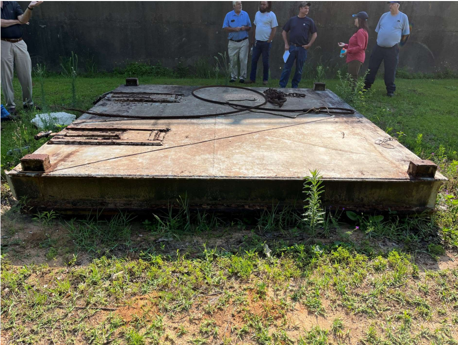
Valve Bulkhead Original Condition
